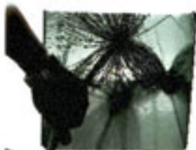
John Matus/Kansas City (Mo.) Star Once air ducts are clean, expect improved energy efficiency in the house.
